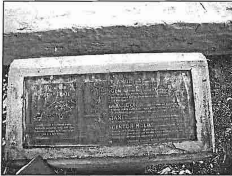
Figure 29. The plinth is also degrading
