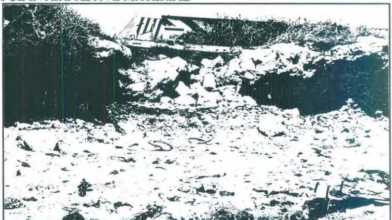
Figure 11. Undercut at inshore end of stone landing, north side (photo: J. Potts, 1993).
