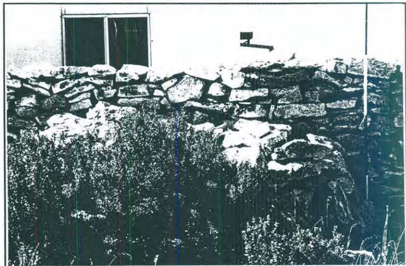
Figure 27. Detail of mid section of south stone wall 1640 HA011; artefacts located in between boulders (photo: M. Stanbury, 1993).
