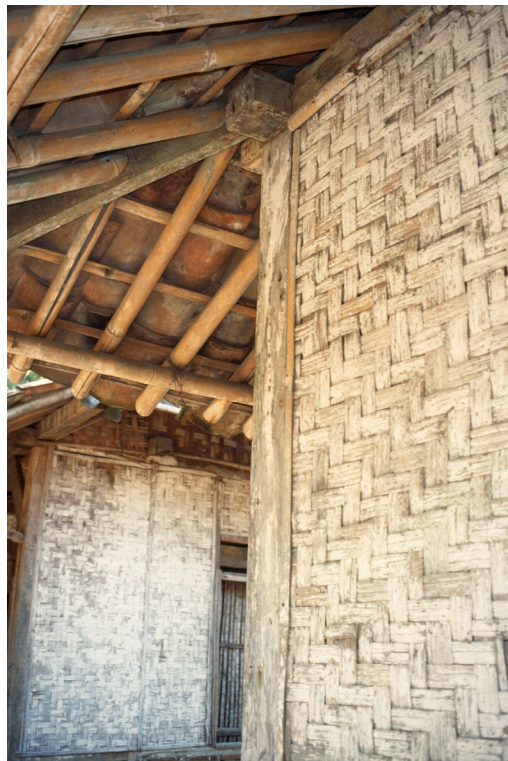
Figure 183: Kampung house with roofing tiles on bamboo battens. Photographed at Batujaya, West Java.
