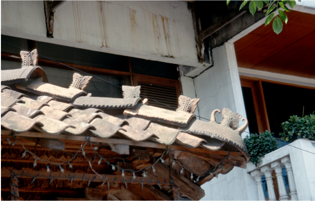
Figure 203: Hip-tiles on the roof of an antique shop in Ciputat Raya in Jakarta.
